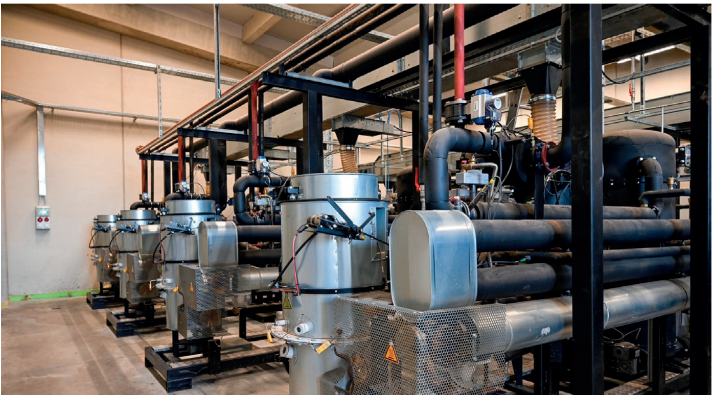
INSTALLED WOOD GASIFIER UNITS
