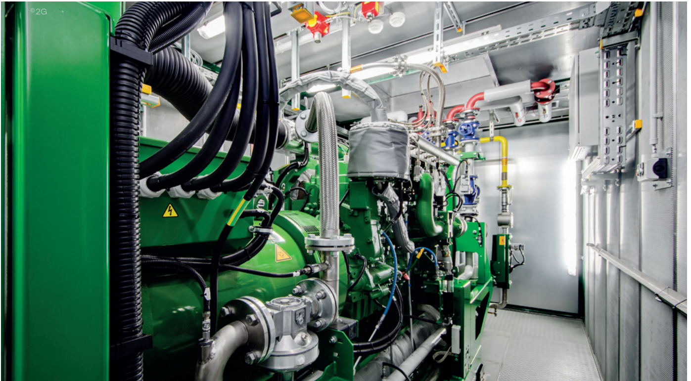
HIGH-PERFORMANCE WOOD GAS CHP PLANT
