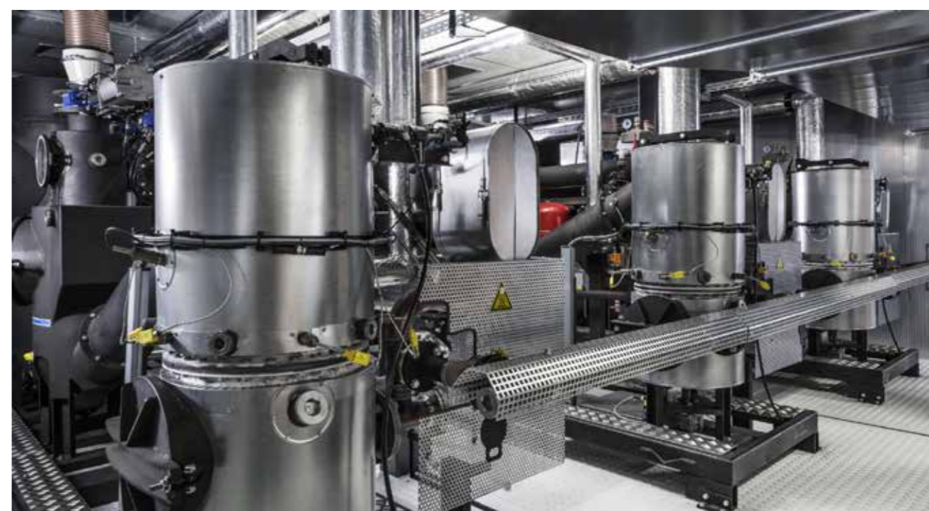
The electrical output is around 150 kWel. The thermal output is around 350 kWth.
