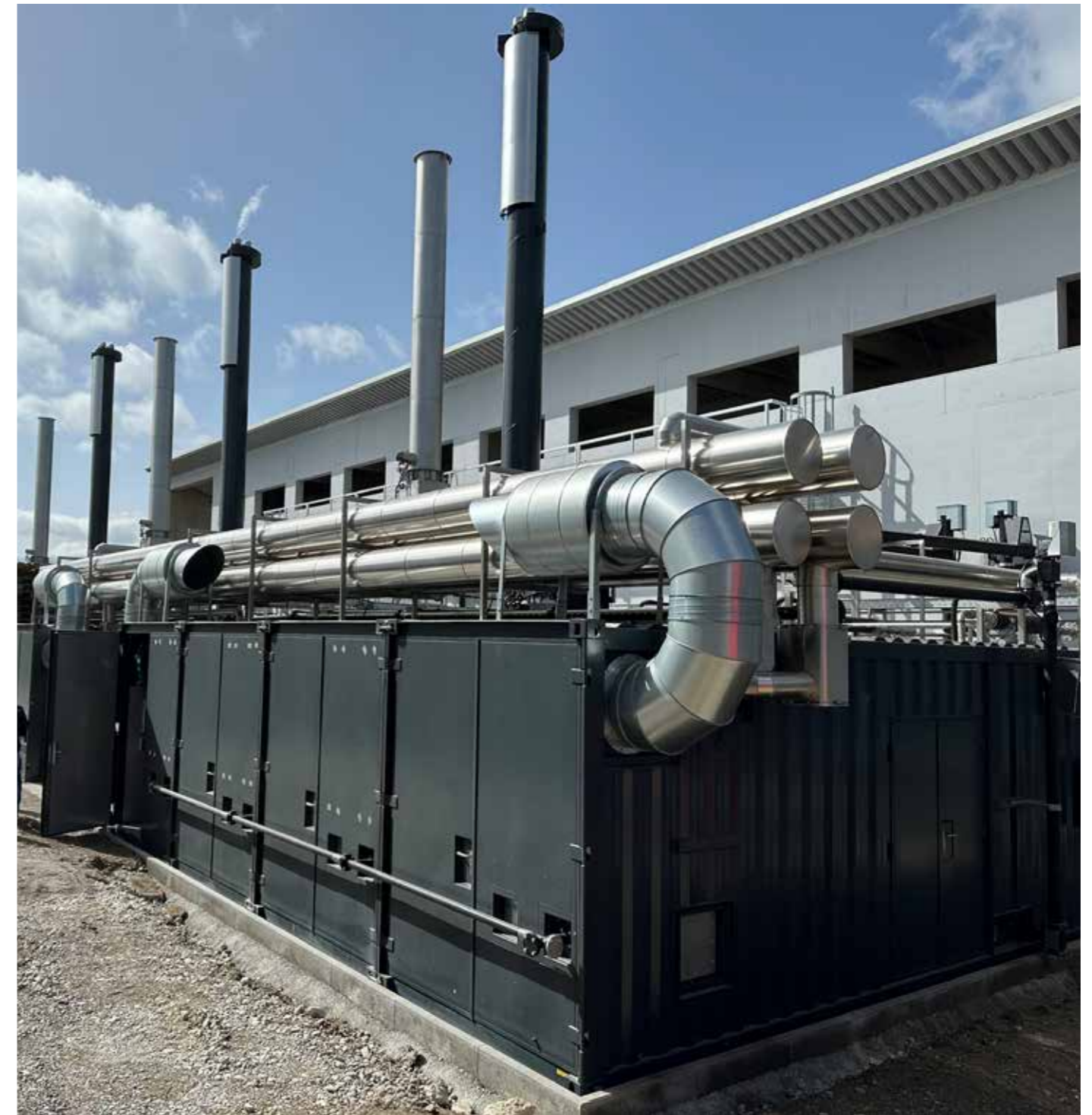
4 x turn key EnergyBlocks with pre-installed gensets.
