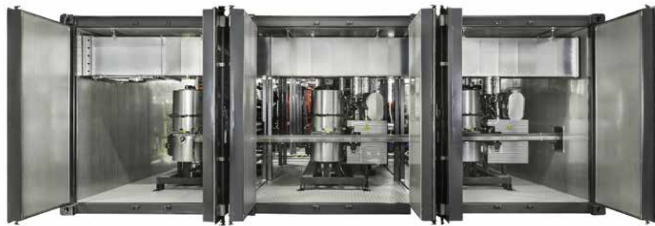
TRIPLE CONTAINER SYSTEM INSTALLED BY FIRST NATIONS (CANADA)
